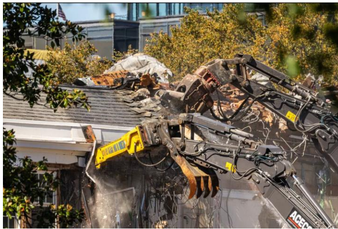
Figure 9 – Demolition of the East Wing of the White House. Alex Kent / The New York Times.
