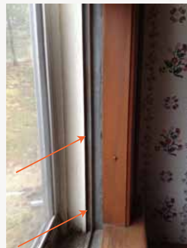
The red arrows indicate metal weather stripping that fits into a routed channel along the sides and bottom of the sash.
