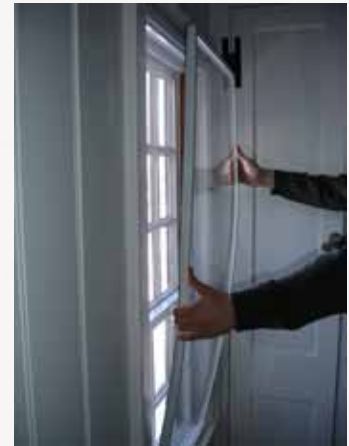
Interior storm panel.
